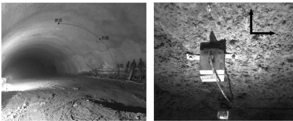
(a) 拱部测点布置 (b) 传感器的安装 (a) Layout of arch measuring points (b) Installation of sensors
