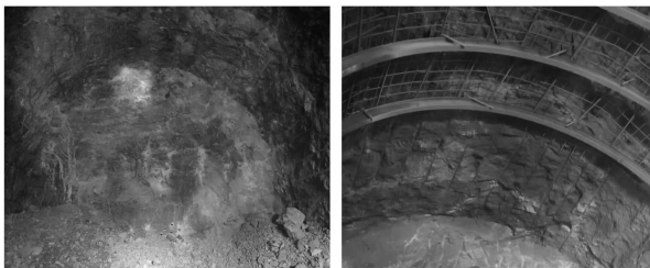
(a) 出渣后整体效果图 (b) 爆后拱顶效果图 (a) Overall effect diagram after slag discharge (b) Post-blast vault effect diagram
