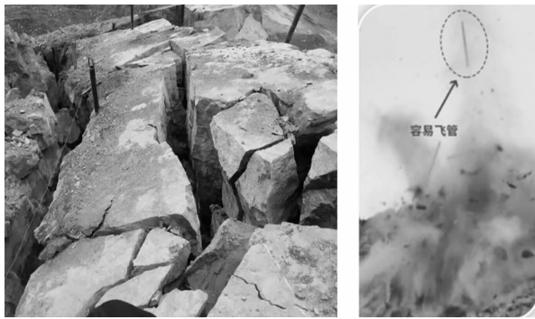
(a) 露在孔外的致裂管 (a) Cracking pipe exposed outside the hole (b) 飞管现象 (b) Flying pipe phenomenon
