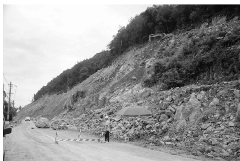
(a) 路面及右侧待开挖边坡 (a) Road surface and right side slope to be excavated
