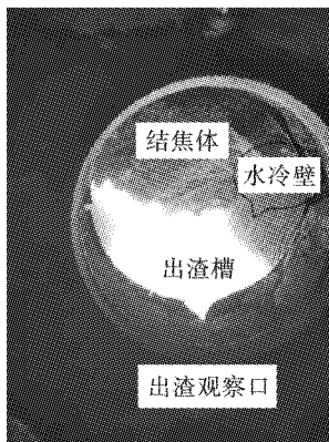
图2 煤粉锅炉结焦环境照片 Fig. 2 Picture of coking environment of pulverized coal furnace
