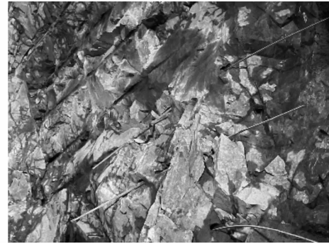
图9 右边墙聚能装置装药拒爆 Fig. 9 Misfire of the shaped charges on the right wall
