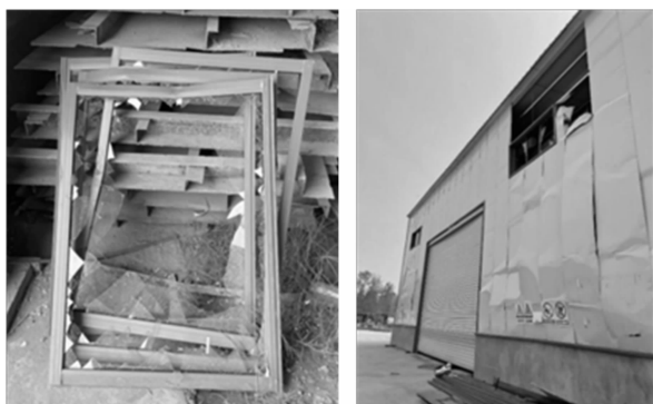
(a) 脱落的窗框 (b) 彩钢房外壁 (a) Dislodged window frames (b) Outer wall of the color steel room
