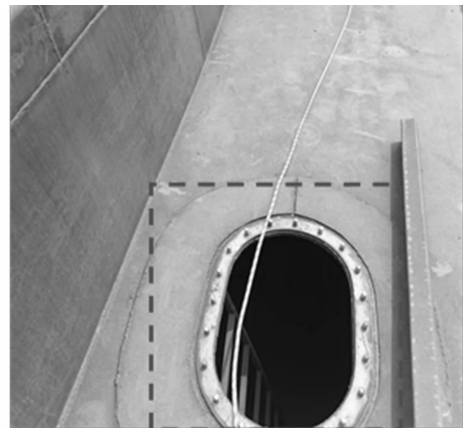
图5 No. 7 空舱主甲板人孔 Fig. 5 The utility hole on the main deck of No. 7 empty cabin
