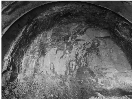
图12 新旧方案隧道成型轮廓对比 Fig. 12 Comparison of formed tunnel contours between new and old schemes
