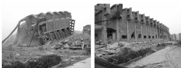
(a) 左侧折叠爆破拆除结果 (a) Folding implosion result of the left part (b) 右侧定向爆破结果 (b) Directional blasting result of the right part
