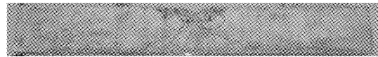
(c) BFRC2 梁破坏形态及裂纹图 (c) Damage pattern and crack diagram of beam BFRC2
