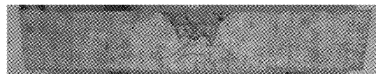
(b) BFRC1 梁破坏形态及裂纹图 (b) Damage pattern and crack diagram of beam BFRC1
