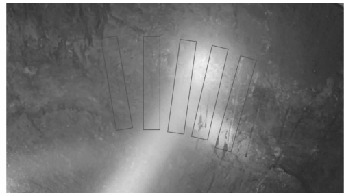
图8 隧道拱顶侧面软弱带排险后形成的圆顺岩壁 Fig. 8 Round rock wall formed after the soft zone on the side of the tunnel vault is removed
