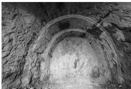
图 8 错台过宽导致超挖较大 Fig. 8 The platform is too wide causing overcut
