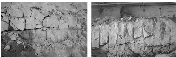
(a) 上游预裂爆破效果 (a) Upstream pre-splitting and blasting effect (b) 下游预裂爆破效果 (b) Downstream pre-splitting and blasting effect
