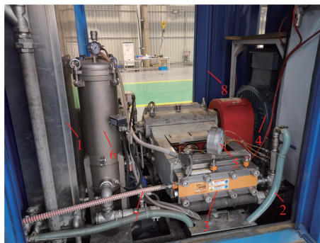
图 14 超高压柱塞泵系统 Fig.14 Ultra-high-pressure plunger pump system
