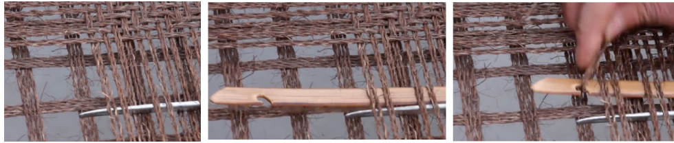
图 20 铁钎“开道”、竹片引棕绳工序实拍 Fig. 20 Photographs of the process of palm rope threading with iron rod and bamboo strip
