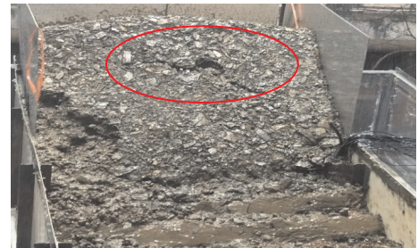
(a) 坡面裂缝
