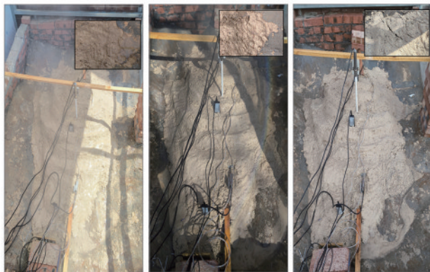
(a) 侵蚀浸润 (b) 破坏加剧 (c) 整体破坏
