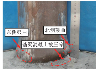
图5 试件H0-1-6的破坏形态 Fig. 5 Failure mode of specimen H0-1-6
