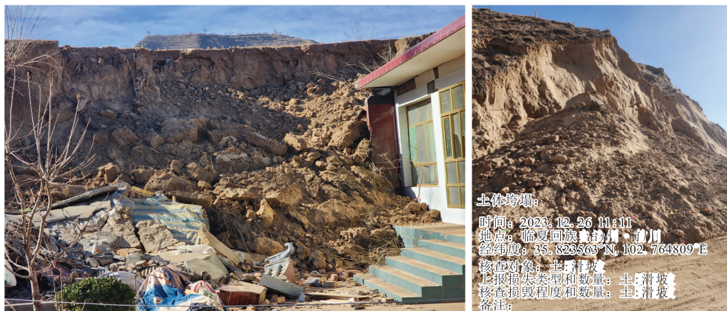
(A)大河家镇切坡边坡滑坡
