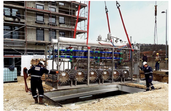
图10 氢能系统在地下能源中心的集中布置 Fig. 10 Centralized arrangement of hydrogen energy systems in underground energy centers
