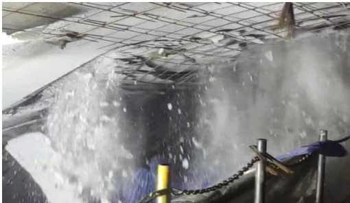
图 16 埋深 300 m 处轻微岩爆灾害现场 Fig. 16 Site of light rock burst at the buried depth of 300 m
