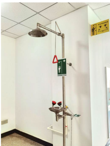
Fig. 3 Emergency spray eye wash device
